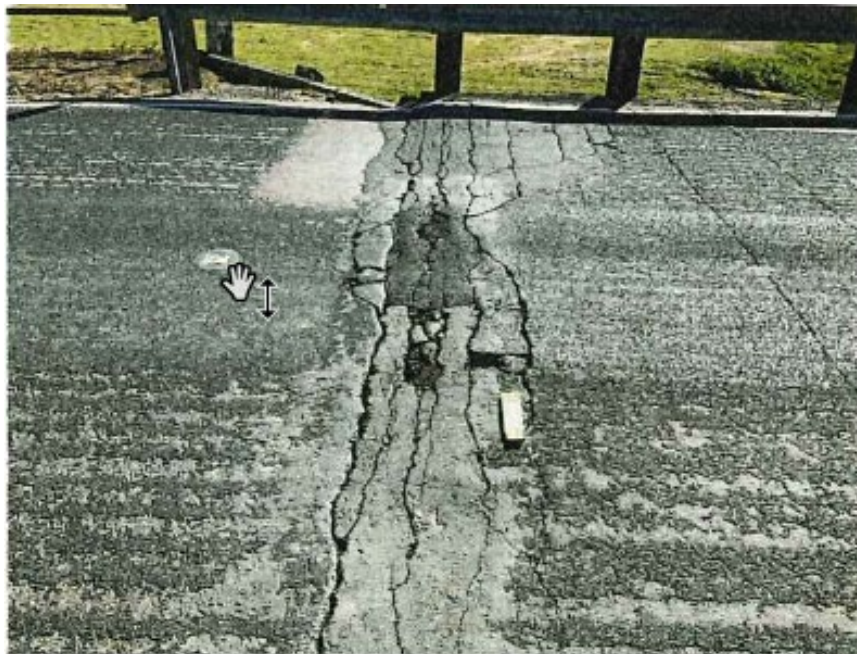
Figure 2. Photo of deck wearing surface deterioration looking at abutment 3 westbound lane.
