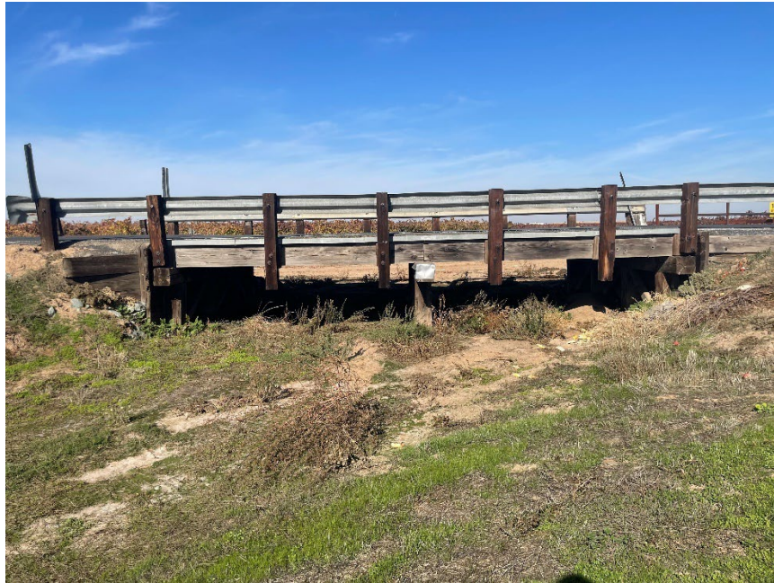
Figure 1. Photo looking north, from downstream, at the right side of the bridge.
