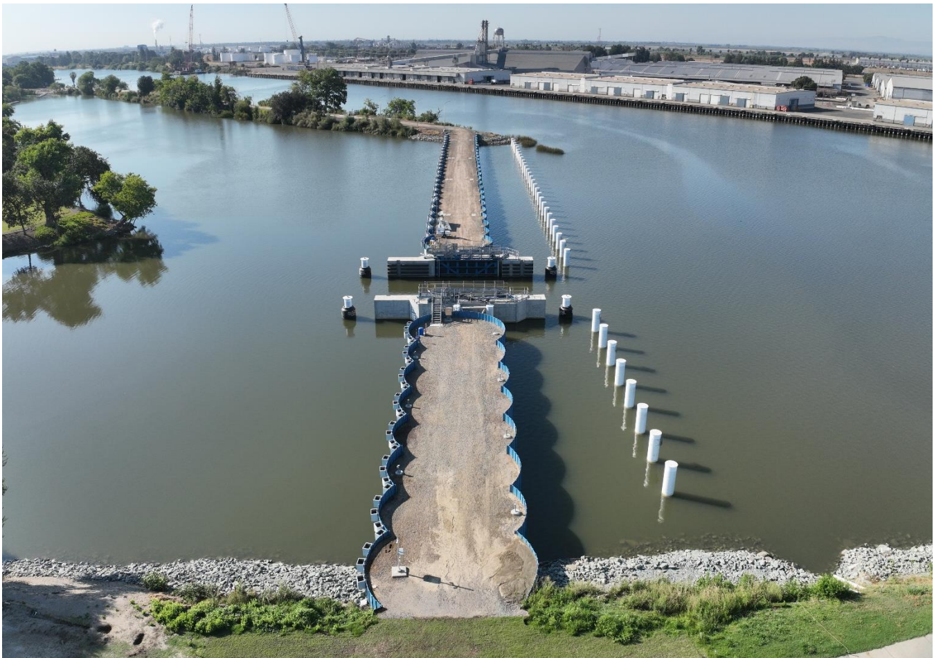
Smith Canal Flood Control Gate, Photo source: San Joaquin Area Flood Control Agency
