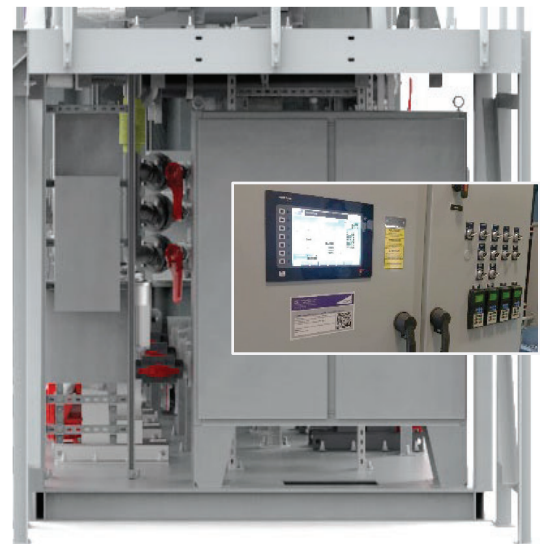
FIGURE 14 – PLC | HMI | MCP
