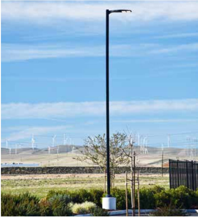
Typical Single-Head Parking Lot Lighting
