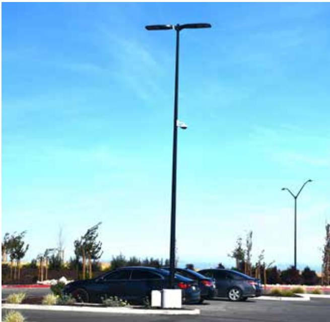
Typical Double-Head Parking Lot Lighting
