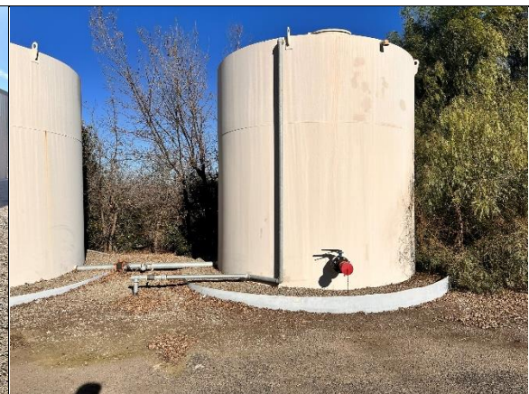
Photograph 57: View of Water Tanks Used for Fire Suppression System.
