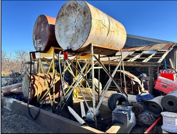
Photograph 1: View of Two, 200-Gallon fuel Aboveground Storage Tanks (ASTs) Located Outside the Shop Area West of Chrisman Road.
