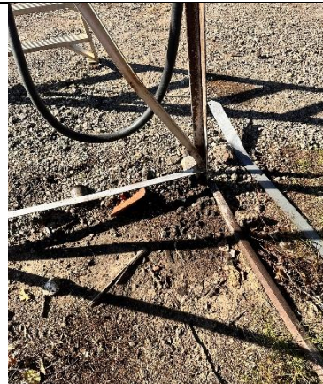
Photograph 112: View of Stained Area Beneath Fueling AST.
