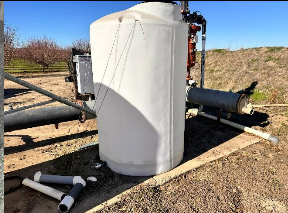
Photograph 64: View of Empty Storage Tank Near Supply Well.
