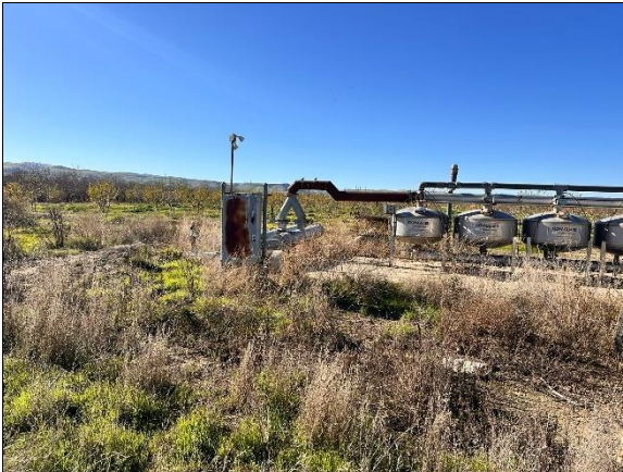
Photograph 117: View of Groundwater Well Filtration System Located Along Northern Boundary.
