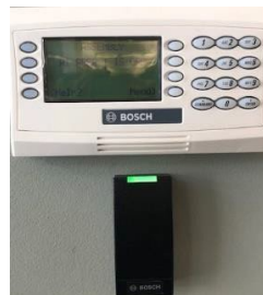
Figure 2. Alarm Keypad and Scanner
