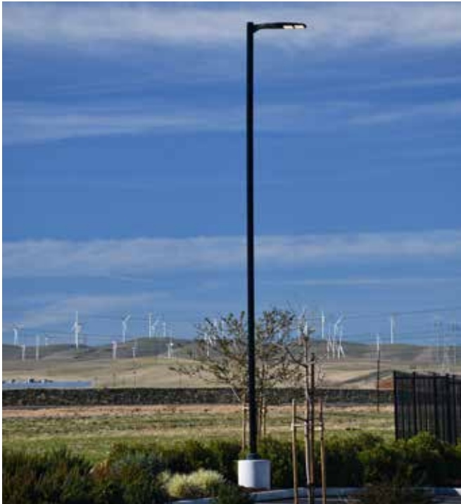
Typical Single-Head Parking Lot Lighting
