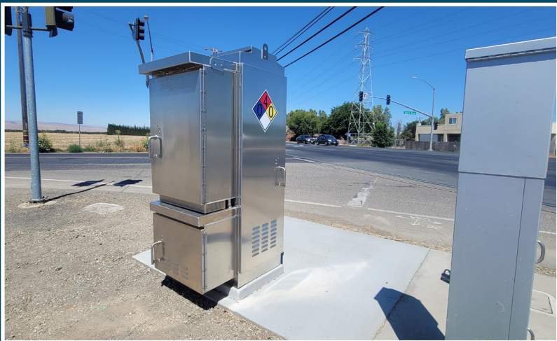
Traffic Signal Power Back Up System
