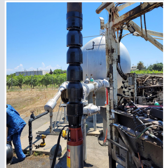
Acampo Well #2 Replacement Pump
