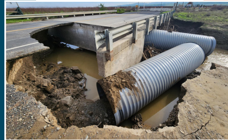
MacArthur Road Bridge Washout
